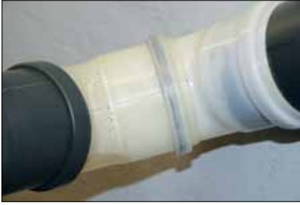
Little heat goes to waste. Here, a test unit exhaust is piped through simple plastic tubing through which condensing water is visible.
